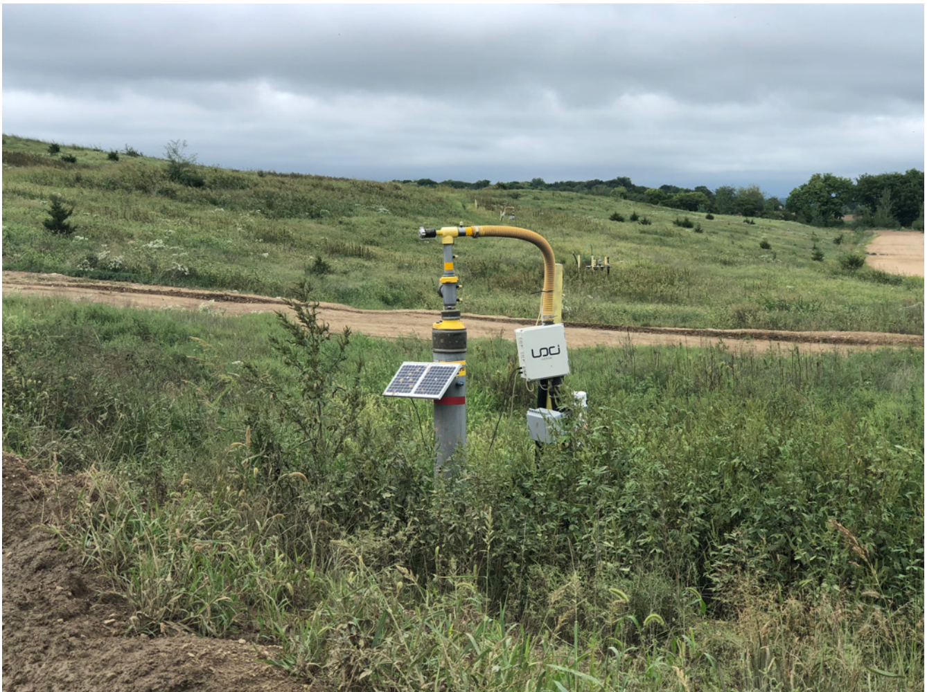
Photo 1: Loci Controller unit on well at the Hamm Landfill in September, 2018.
