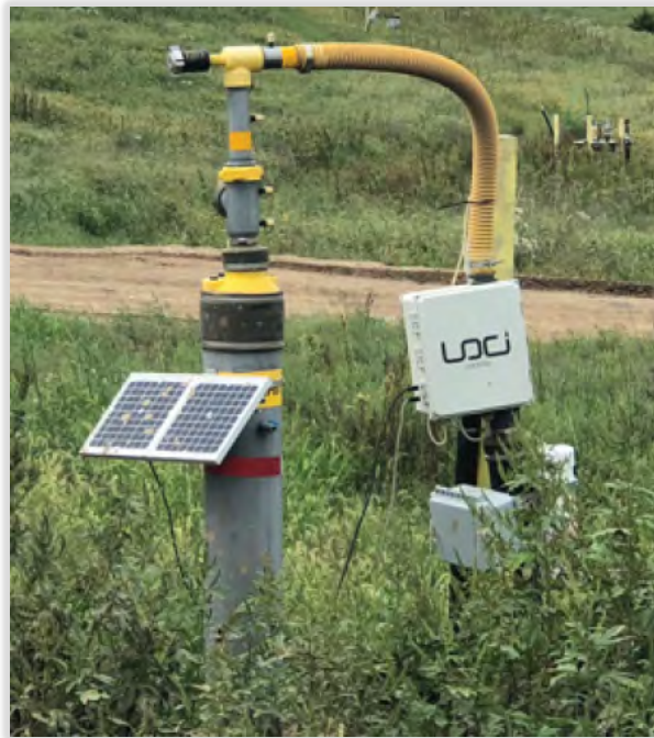
Figure 9. View of Vertical Landfill Gas Collection Well Equipped with the Loci System (image source: Loci Controls).
